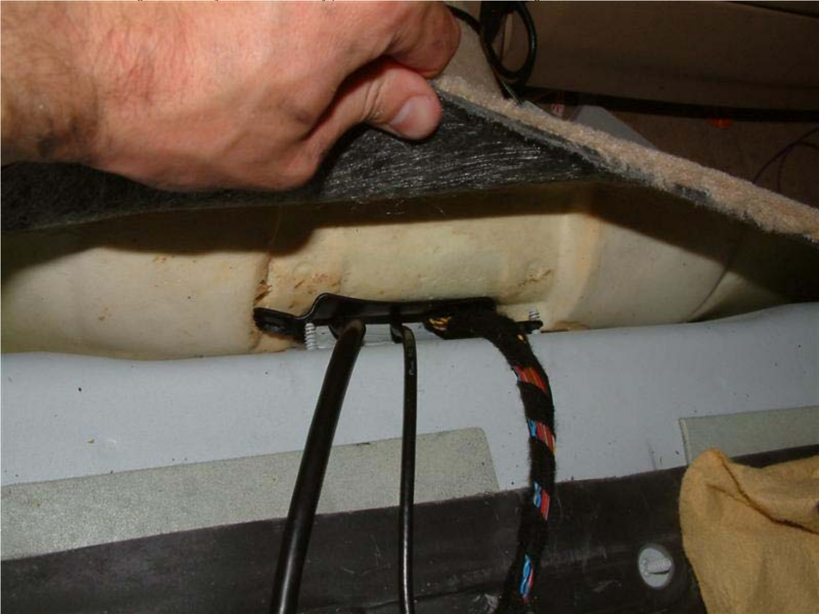
Once the wires are through the tunnel you can find an easy path to the center console for running the wires
